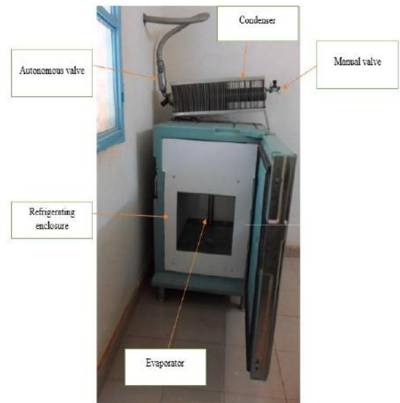
Fig.4. Detailed photograph of the condenser and the refrigerating enclosure
